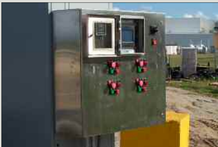
Ensuring your plant's optimum Dissolved Oxygen (DO) at minimal energy consumption.
